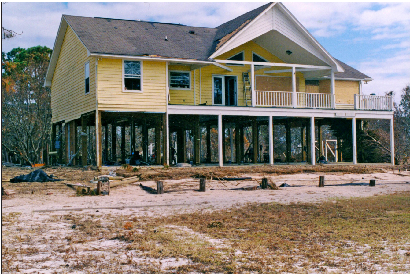
Figure 28: Home elevated above the BFE in Zone AE showing successful failure of breakaway walls.
